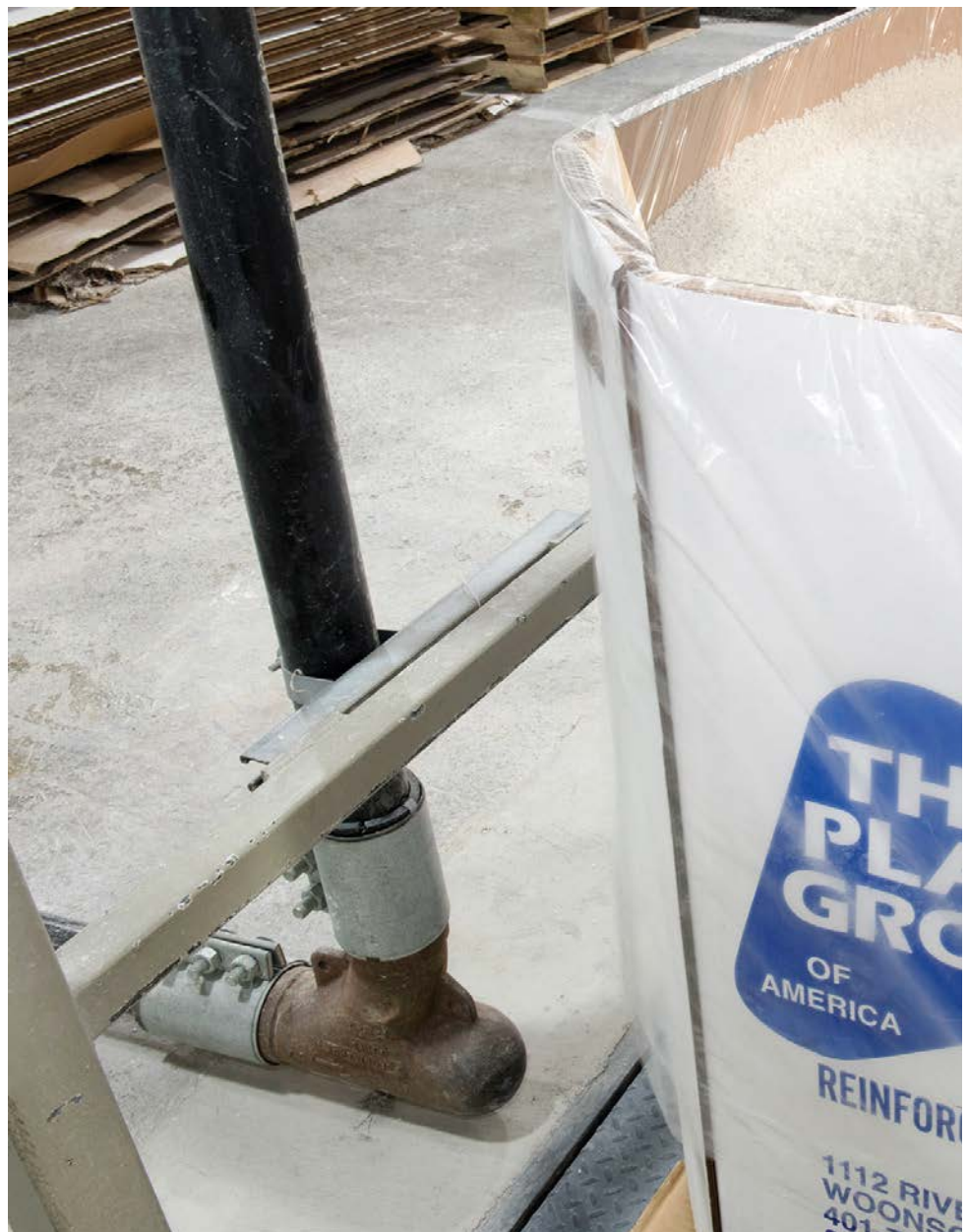
The Plastics Group replaced conventional sweep elbows with HammerTek deflection elbows, none of which has needed replacing. By preventing material impact with the elbow wall, the company has prevented elbow wear, the generation of fines and the frictional heat that previously caused the formation of angel hair and streamers.
